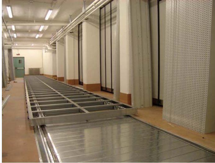
(MOBILE BAYS WITH WOODEN PLATFORM)
